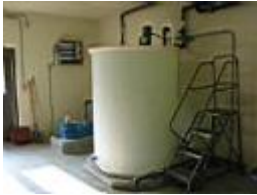
Polymer Mixing Tank.JPG
