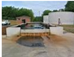
Vacuum Bed, Thickeners & Control Building.JPG
